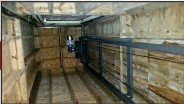
Drum Above Installation
